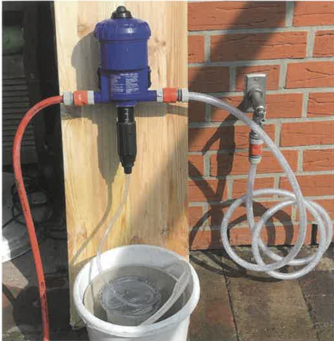
Simple installation of a Dosatron Proportional Doser. (Photo: Jens Voigt)
